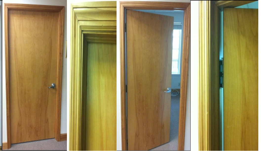
Unprotected -Push Side Door (framed on left) Door Closed and Open View
